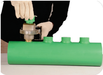
Heat up the Weld-in Saddle and ID of the pipe with proper Dies
